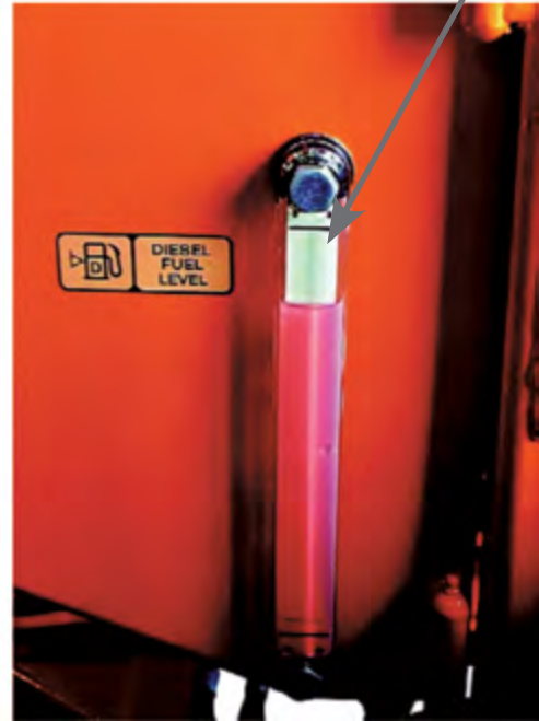
Diesel fuel level
